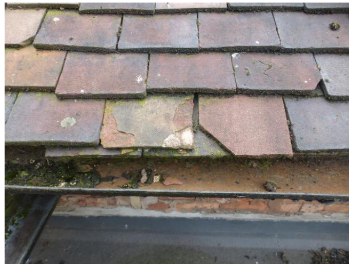
Cast iron gutter and broken and spalling roof tiles
