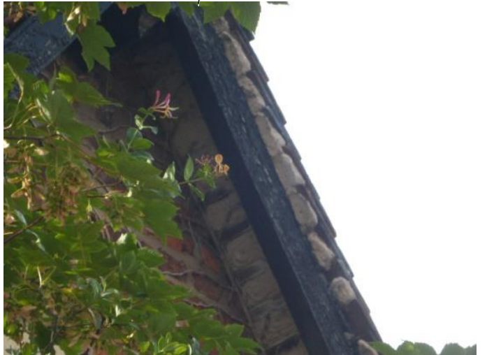
The gable end roof overhang is to be under-boarded using 18mm T & G boards painted black and an under-cloak board is to be provided under the overhanging edge tiles to allow pointing to the tile edge
