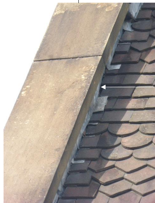
Existing stone coping blocks are to be removed to allow lead flashings to be replaced. The copings are to be replaced using stainless steel restraint angles in the joints as per SE detail
