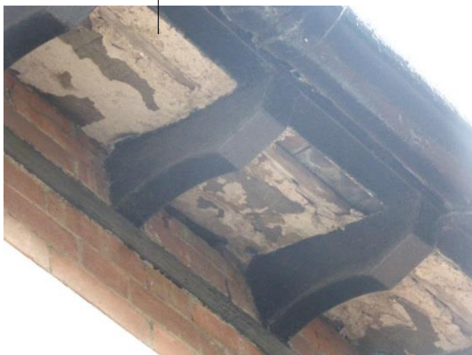
The eaves overhang soffit is to be removed and the soffit is to be boarded with 18mm T & G boards, painted black
